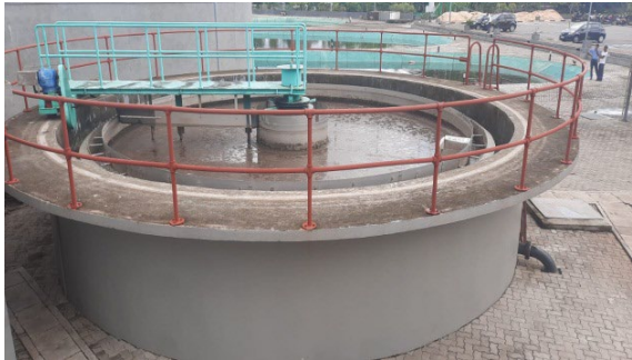
Defense Headquarters - Akuregoda Activated Sludge Extended Aeration Treatment System + Maturation Ponds 1200 m 3 /day
