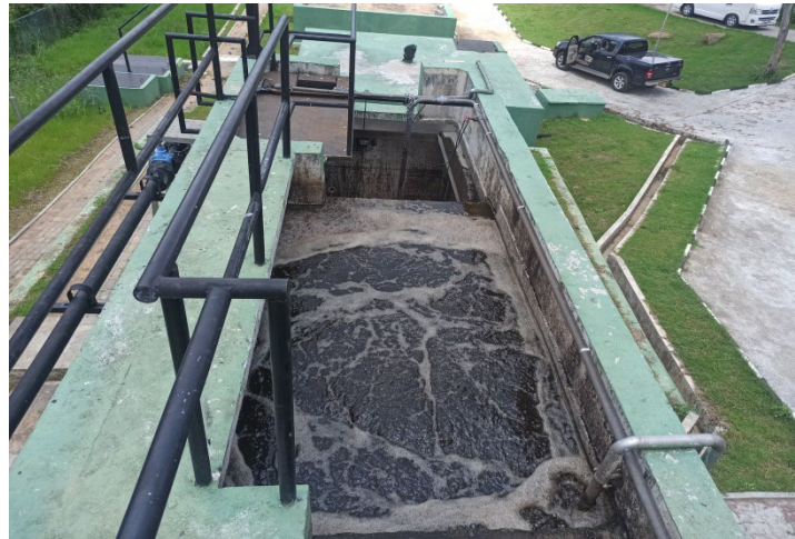
Thalawakele Faecal Sludge Treatment Plant (25m 3 /Day)
