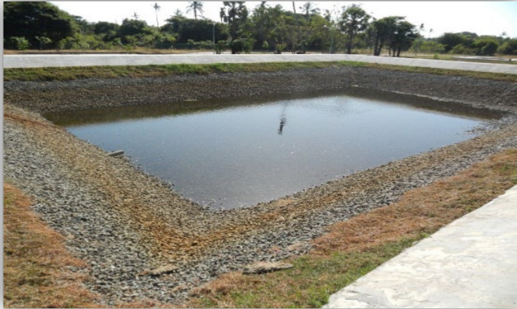
Chilaw Faecal Sludge Treatment Plant (25m 3 /day)
