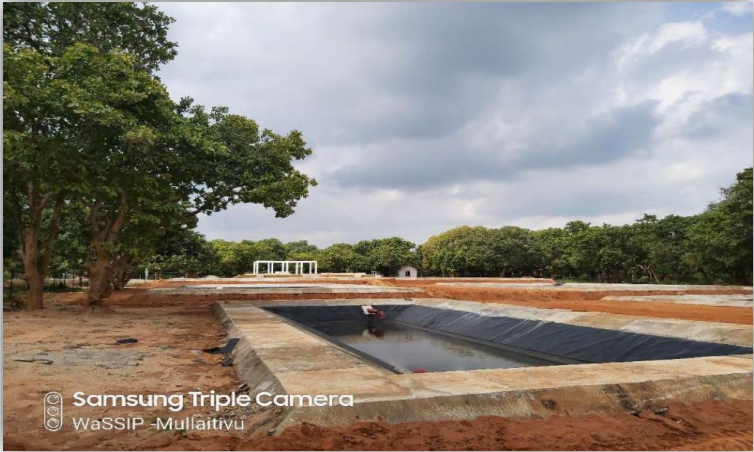
Mulathivu Faecal Sludge Treatment Plant (25m 3 /day)
