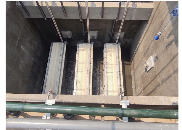
Peliyagoda Fish Market UASB+ MBR System
