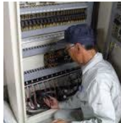
Check control panel
