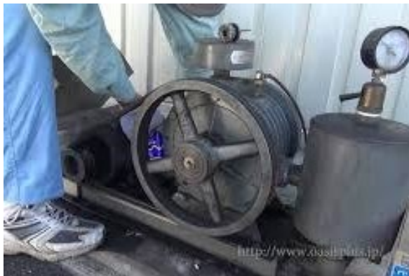
Check operation status of blower
