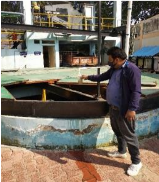
SEWAGE PUMPING STATION
